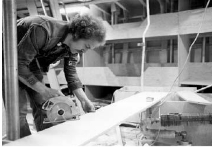
Working seven days a week, we built bunks and galleys for 32 crew members in what had been an empty shell of a ship. By the time we set sail the M.V. James Bay was nicely equipped. Photo: Rex Weyler
